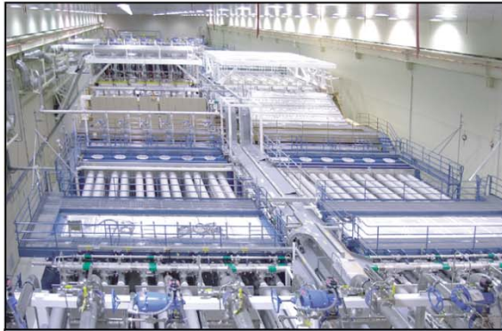
First four laser beams of NIF installed for commissioning beginning in November 2002
